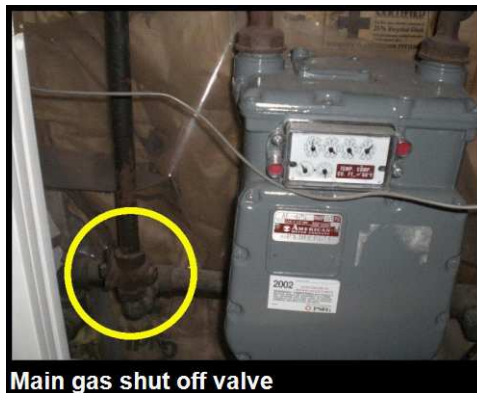
Main gas shut off valve
