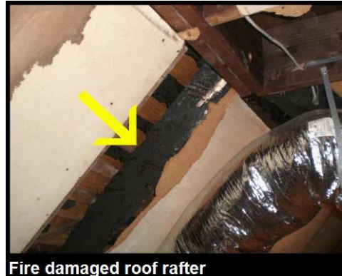
Fire damaged roof rafter
