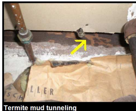
Termite mud tunneling
