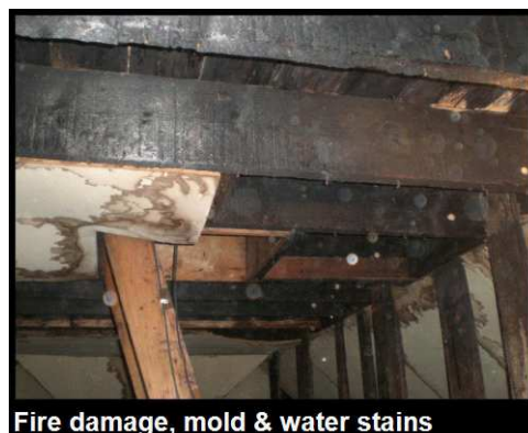
Fire damage, mold and water stains
